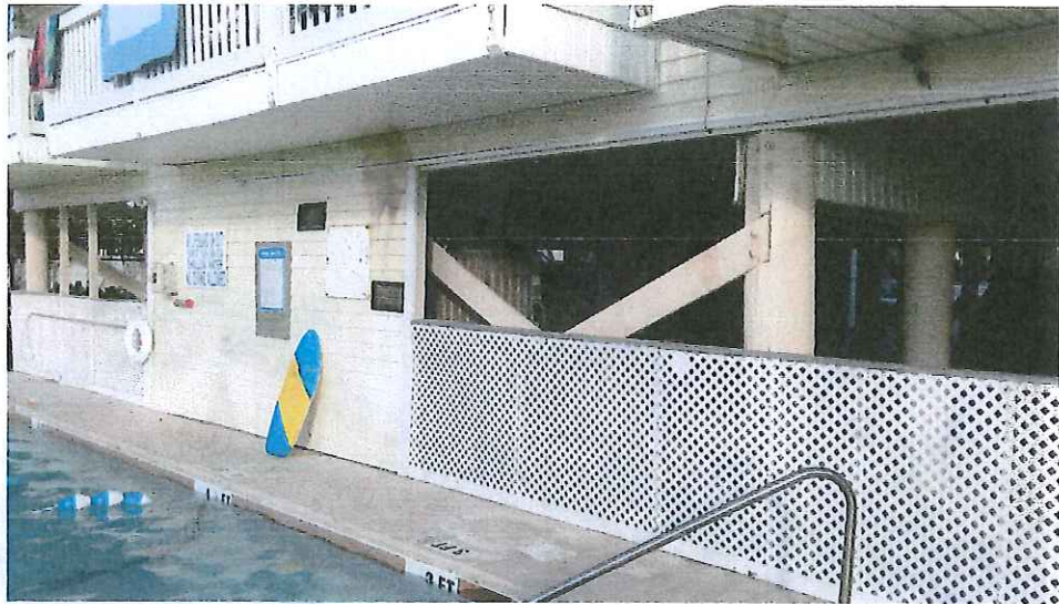
Pool Equipment Enclosure August 17, 2015
