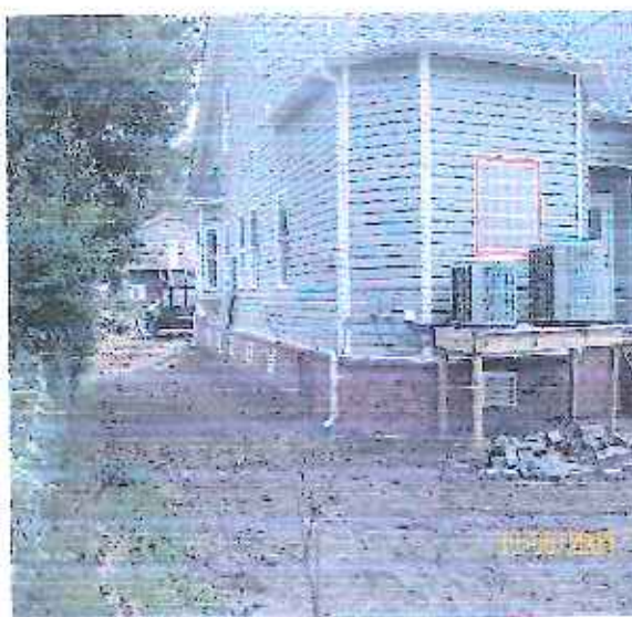
RIGHT SIDE REAR HVAC PLATFORM
