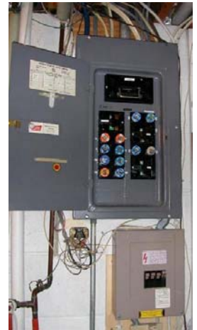
Mark your fuse or breaker box to show the circuits to the floodable areas. Turning off the power to these areas can reduce property damage and save lives.
